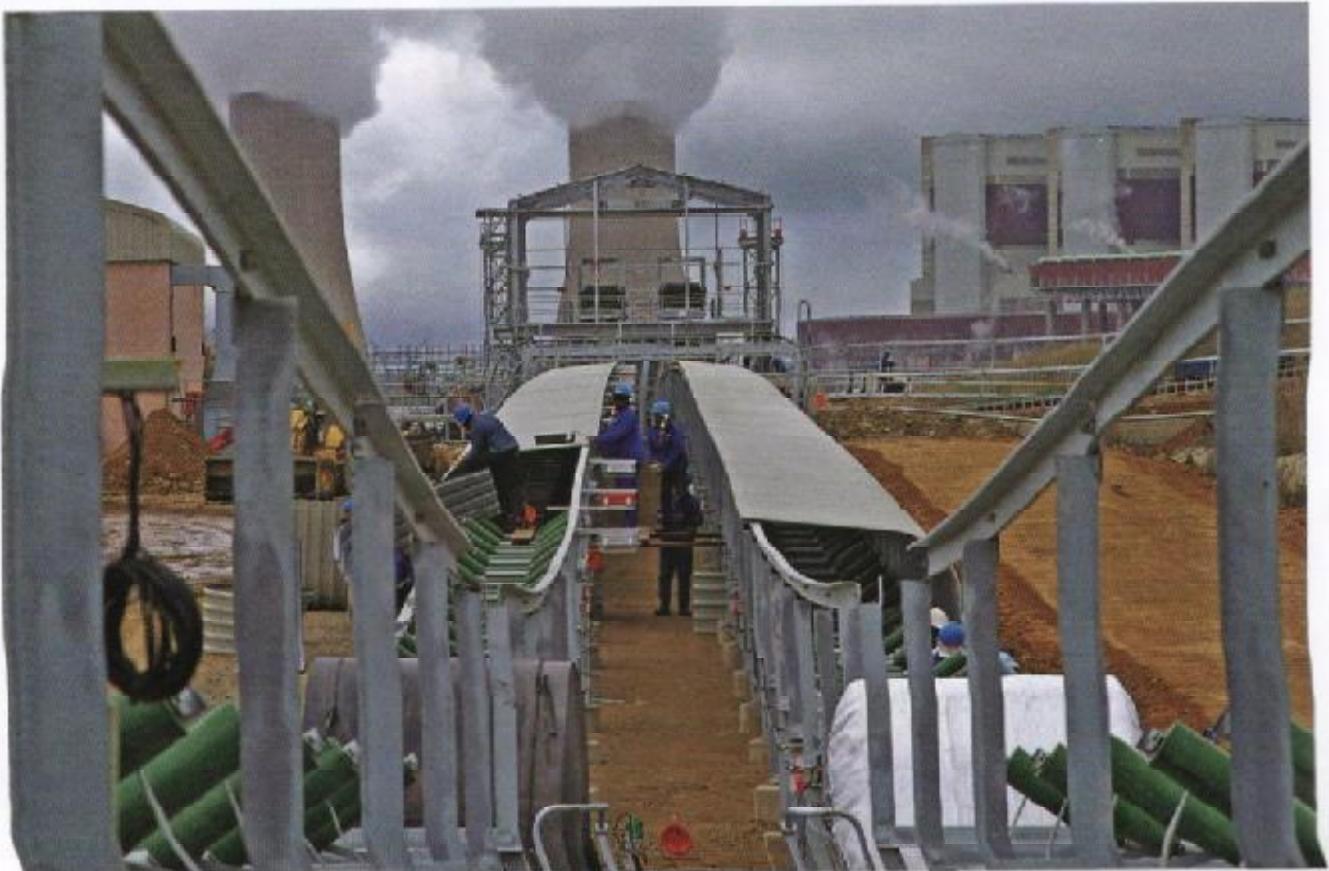
A conveyor system installed at a power station
