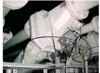
Silo Discharge Arrangement with Flow Control Valve ▼
