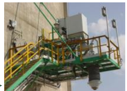
► Emergency Truck Loading facility
