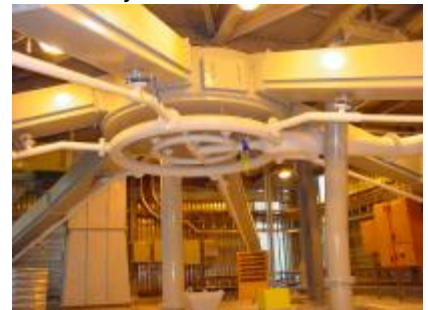
Silo Discharge System
